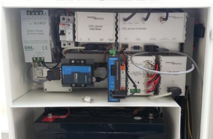
Fig. 2: Example LOG_aLevel housing with different modules. Visible on the lower part is the separate compartment for a buffer battery.
